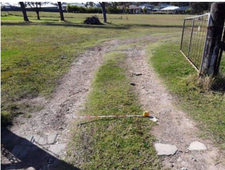
Photo 15 Exposure within vehicle track
