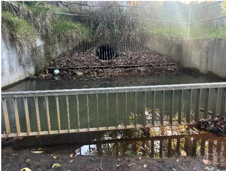
Photo 40: Culvert inlet that drains the Wilton Close reserve
