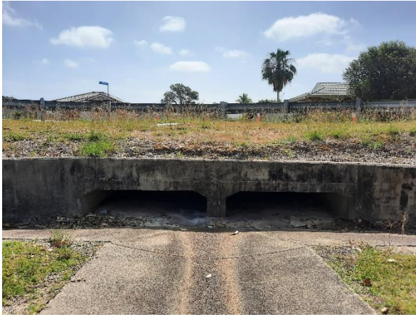
Photo 24: Vermont Place Branch crossing Myles Avenue
