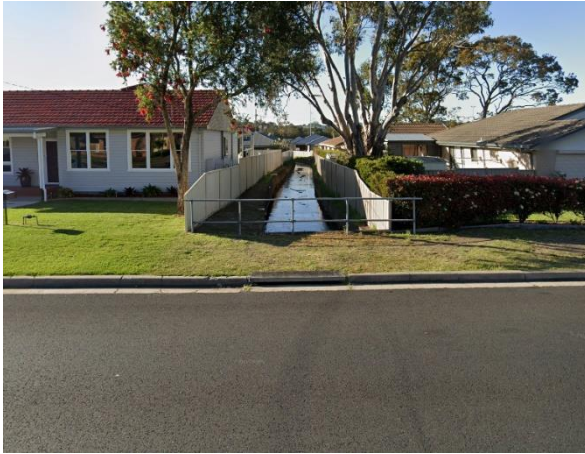
Photo 21: Concrete-lined open channel downstream of Medcalf Street ( Google Street View )
